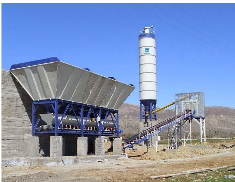
Fig: Dry Mix Concrete Plant
