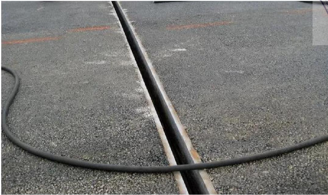
Expansion Joint in Pavement
